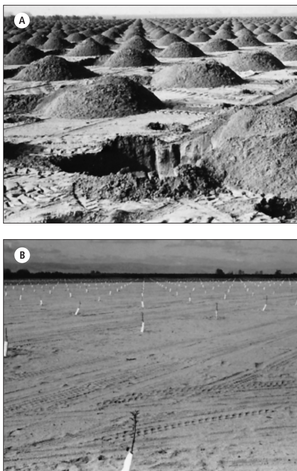
Figure 6.22 Refilled backhoe pits (A) have been found to stimulate growth of young trees, particularly in sandy and stratified soils (B). These pictures were taken 2 months apart.
