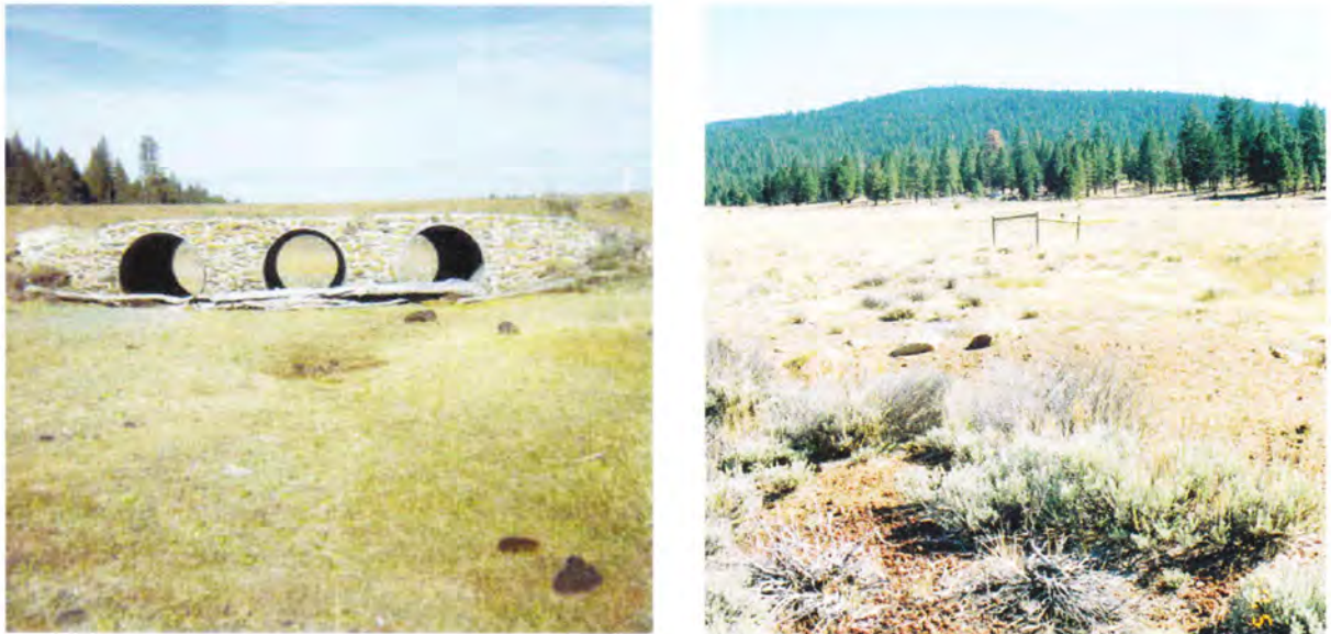
Figure 20. Left, culverts across Pine Creek from Harvey Valley Road crossing, 1976. Right, all road fill removed circa 1988, channel unimpeded and allows for fish passage, 2005.
