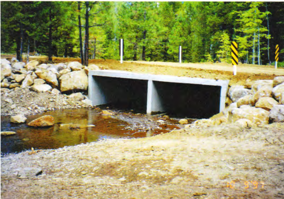
Figure 15. Top, corrugated metal pipe culverts in the early 1990's. Bottom, concrete box culverts to allow for fish migration and pass higher stream flows, 1997.
