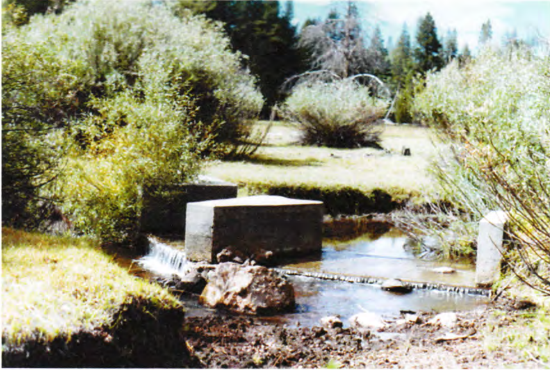
Figure 13a. Splitter structure (1978) downstream of confluence of Pine Creek and Bogard Spring Creek.
