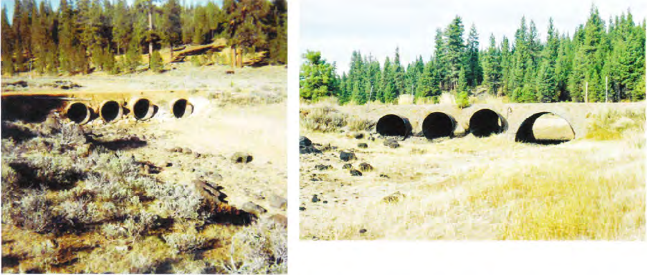
Figure 11. Camp 10 Road Culverts. Left 1976, looking downstream. Right, 2005, looking downstream. Note largest culvert on far right showing low flow, below grade channel.
