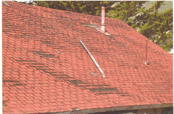
Photo by Stephen Quarles Worn out shingles lose their effectiveness as both fire and moisture resistant materials. Roof coverings must be replaced once they have reached the end of their useful service life.
