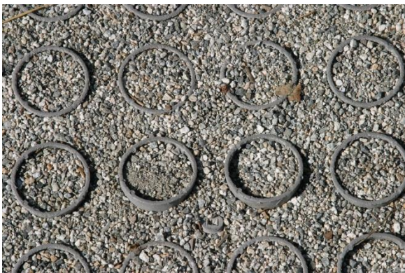
A grid of rubber rings helps stabilize gravel in this parking area.
