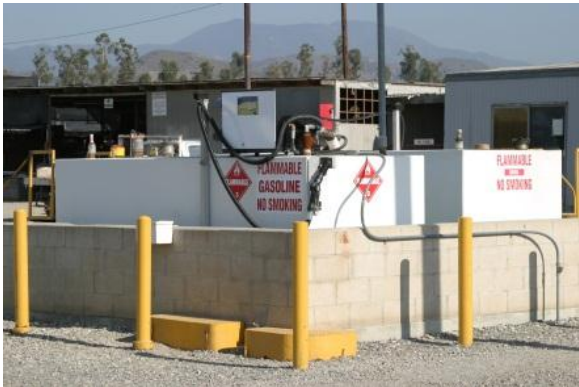
Provide secondary containment for fuel tanks.
