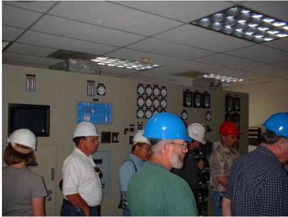
Visitors to the Mt. Lassen Power boiler control room, Westwood, California. July 17, 2003. John Stewart
