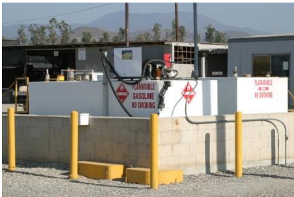
Provide secondary containment for fuel tanks.
