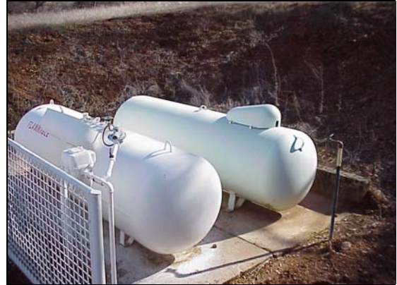
250 Gallon Residential Propane Tanks Photograph Courtesy of Sierra Foothill REC
