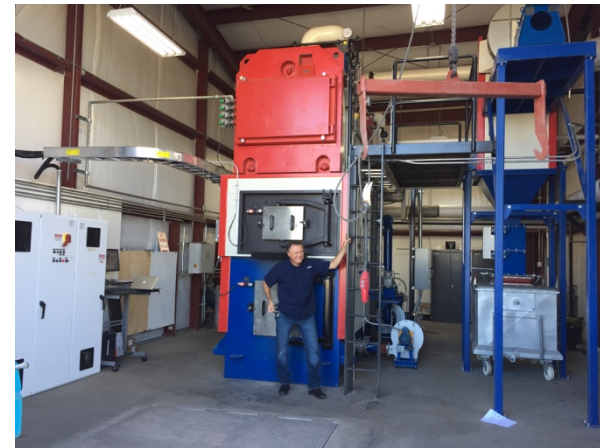
Facility Services Director touring system in Burns
