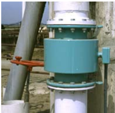
Figure 2. Magnetic flowmeter. Photo: Lawrence J. Schwankl.
