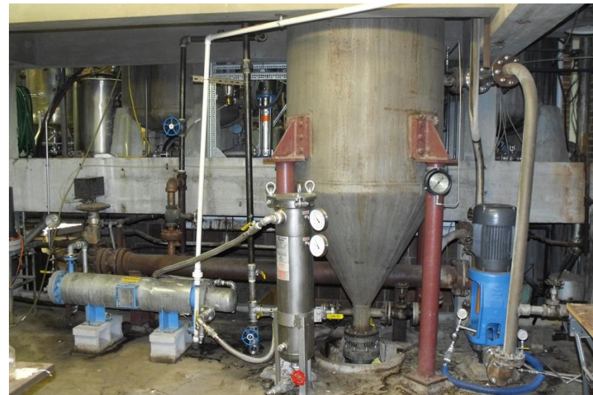
Pilot Extraction System, SUNY ESF
