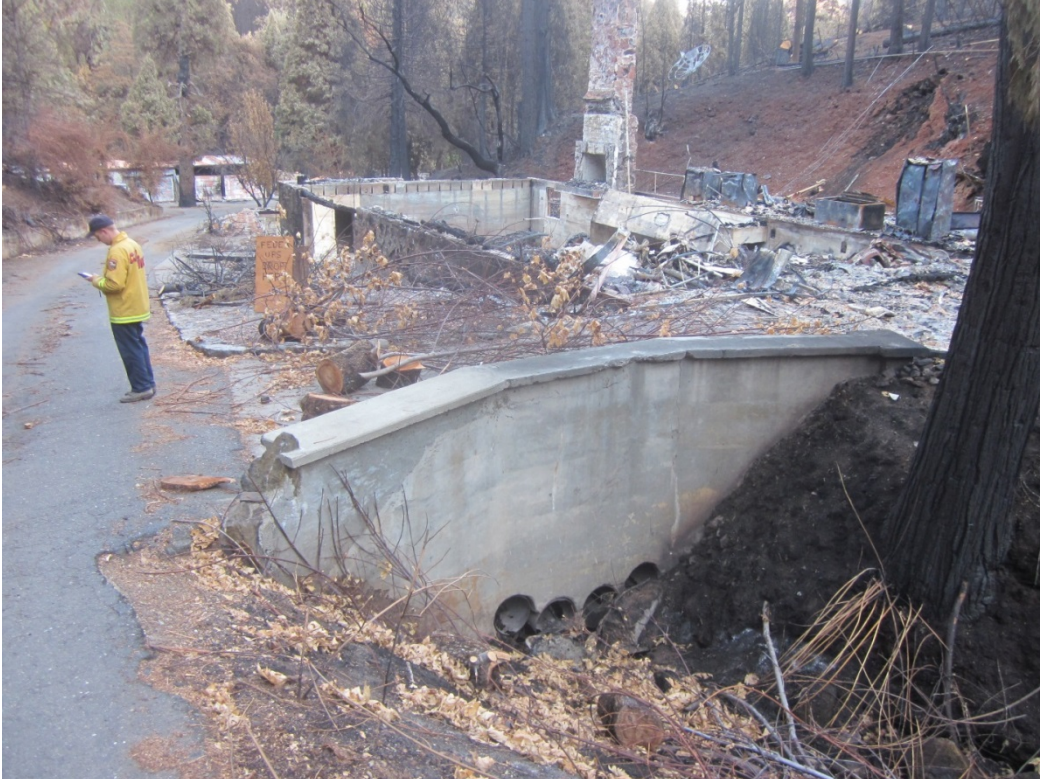
Burned residence constructed within a watercourse. Culverts constructed under the residence may experience increased flows, including sediment, woody debris and ash.
