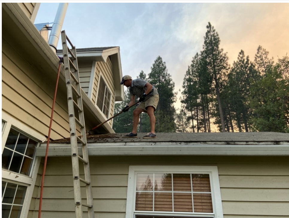
Don't forget to clean your roofs and gutters of any moss, vegetative debris, or leaf litter. Here the author wishes he did this in May rather than waiting until August with wildfire smoke looming in the background.
