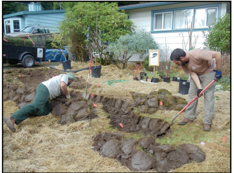
To keep weeds down in the new raingarden, lawns or other pre-existing landscape plants may have to be let go, sheet mulched, or dug up.
