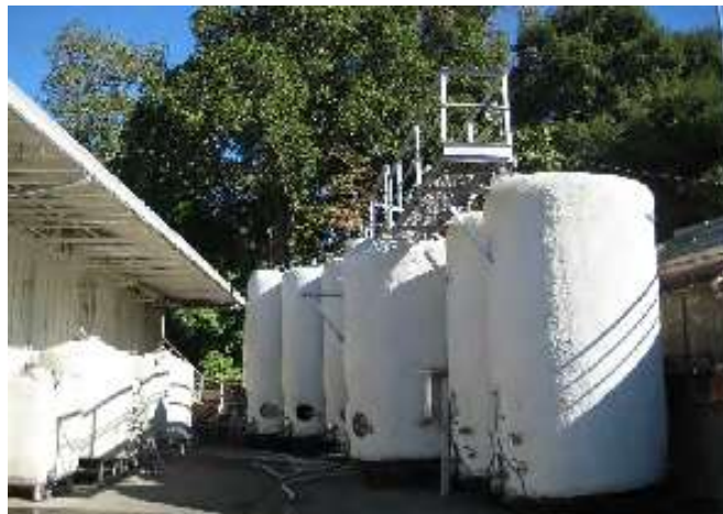
Insulating outdoor tanks reduces tank refrigeration and energy costs, while helping to maintain a consistent temperature for better wine quality.
