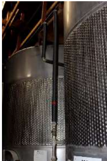
Efficiency improvements to the refrigeration system can include insulating glycol lines.
