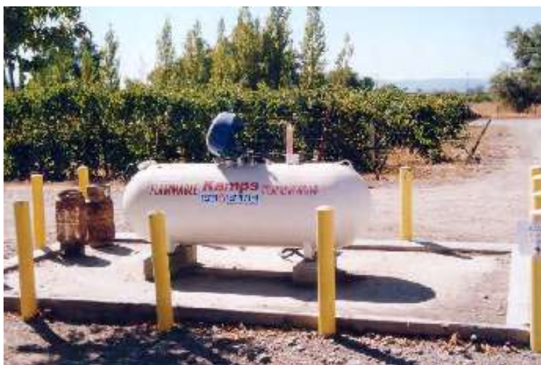
A concrete-padded fueling area along with training employees in fuel handling, spill prevention, control, and clean-up are best practices for aboveground storage tanks.
