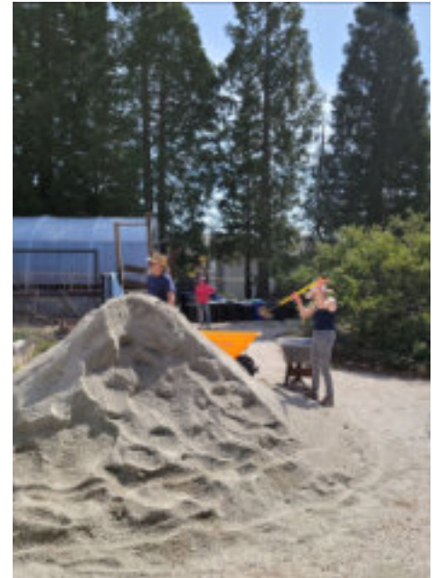
Crushed gravel being spread on walkways at our Demo Garden. Photo by Ann Wright.
