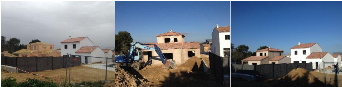
Figure 20. New homes being built in Luyes. Only the roof joists are flammable.
